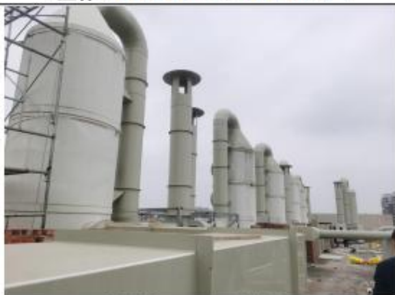
排气筒及活性炭措施 1 (坐标: E110°28'11", N19°59'32")
