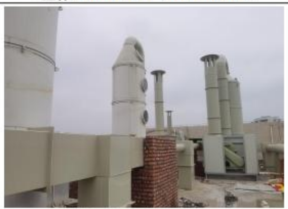
排气筒及活性炭措施 2 (坐标: E110°28'11", N19°59'32")
